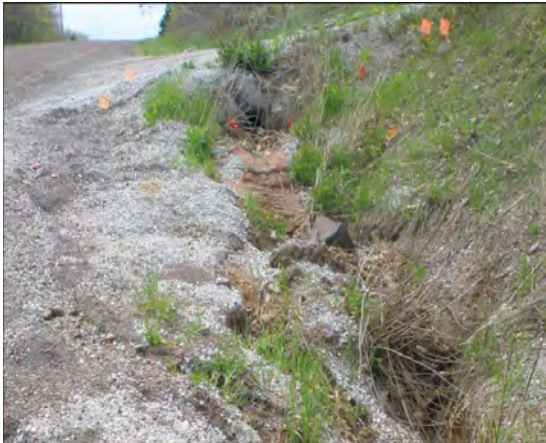
Vulnerable clearing, drainage and erosion
